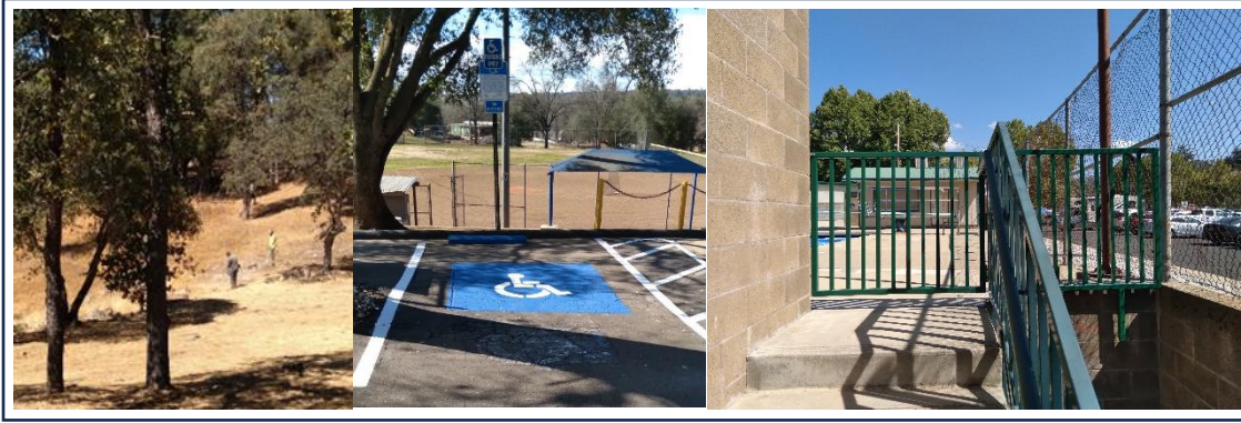
Brush clearing, parking lot painting, and installation of a new gate at the Tuolumne pool.
